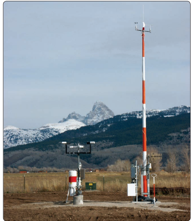
Figure 1-11. AWSS installation at Driggs-Reed, Idaho.
